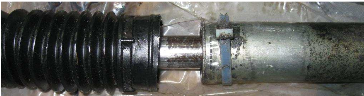
NOT GOOD - Rusty rack
